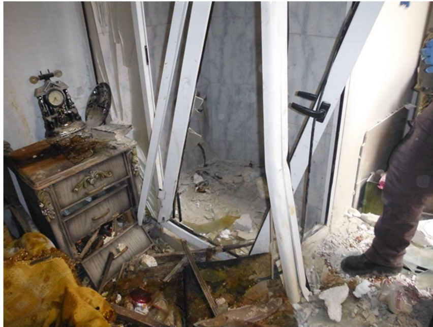
FIGURE 50: PICTURE OF THE DAMAGED SHOWER UNIT. THE DAMAGE IS LIKELY CAUSED BY PARTS OF THE CYLINDER'S ASSEMBLY (SOURCE: FFM)
