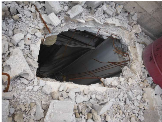
FIGURE 31: CRATER IN THE ROOF AT LOCATION 4, AS SEEN FROM ABOVE.
