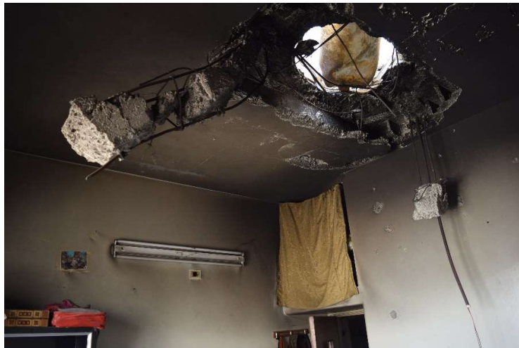
FIGURE 36: FIGURE X: DEFORMATION OF THE STEEL REBARS IN THE CONCRETE TOWARDS THE INTERIOR OF THE BUILDING. (SOURCE: FFM)
