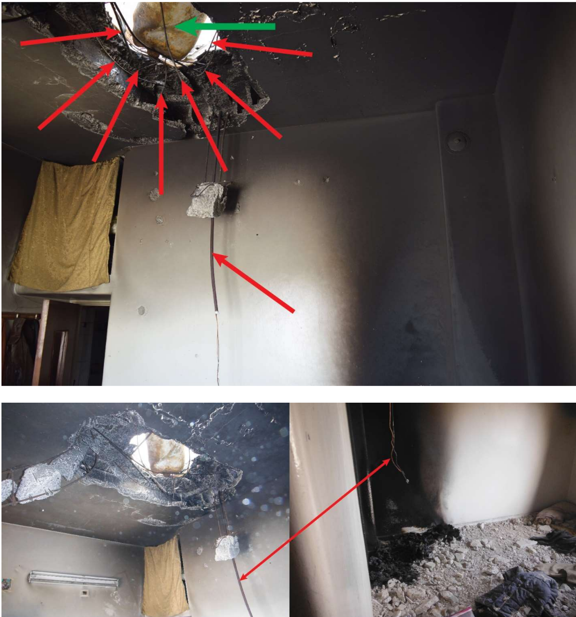
FIGURE 11: VISIBLE CRATER ON THE ROOFTOP OF LOCATION 2 PHOTOGRAPHED FROM THE ROOM DIRECTLY BELOW. PART OF THE YELLOW INDUSTRIAL CYLINDER (MARKED WITH A GREEN ARROW) AND DEPOSITS OF BLACKENING SOOT ON BOTH THE CEILING AND THE WALLS ARE VISIBLE. NO FRAGMENTATION DAMAGE PATTERN CONSISTENT WITH EXPLOSION IS VISIBLE ON THE WALLS.
